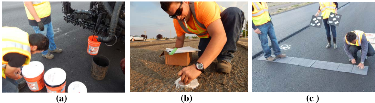
Figure 2.3. Experiments conducted to evaluate tack coat application methods and procedures (a) Emulsion sampling for lab testing (b) Sand patch texture measurements (c) Application rate measurement
