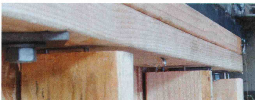
Fig. C12. Top plate separation from the studs.
