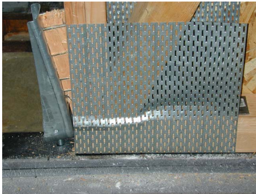
Fig. B22. Failure of the hold-down and buckling of the metal truss plate.
