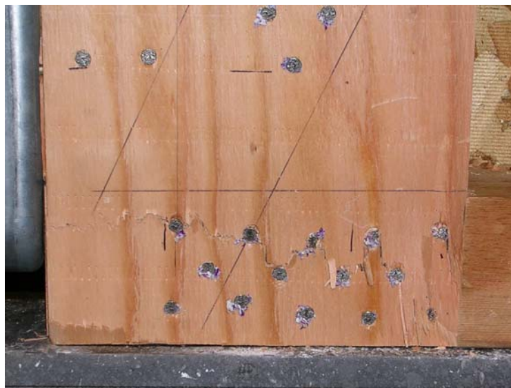
Fig. B22. Plywood gusset plate failure at bottom corner of wall.
