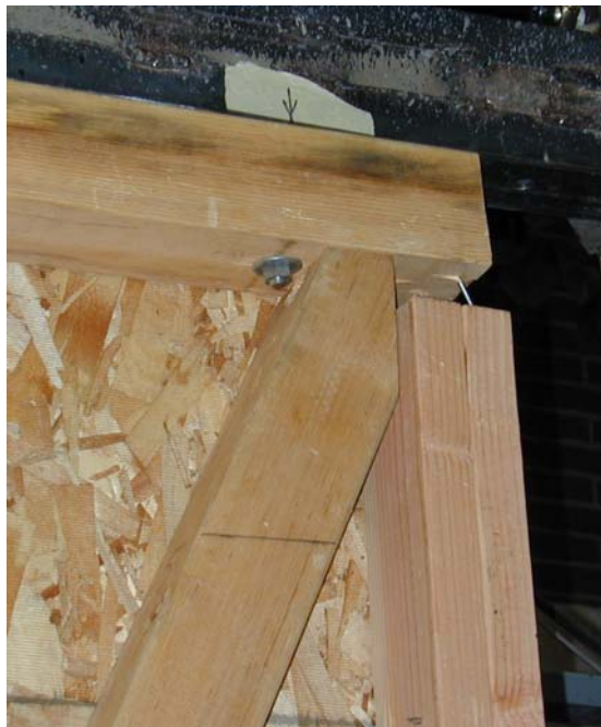
Fig. B20. Braced shearwall top-plate and brace separation.
