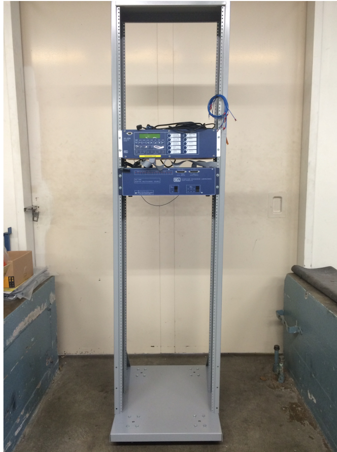
Figure 4.6: A full set of hardware devices for the power system protection laboratory.
