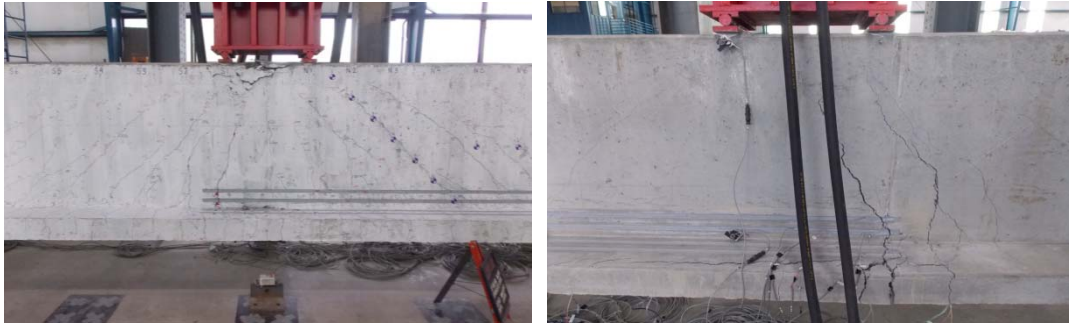
Figure A.57 – Specimen IT.45.Ld3(6).SS front and back failure photographs
