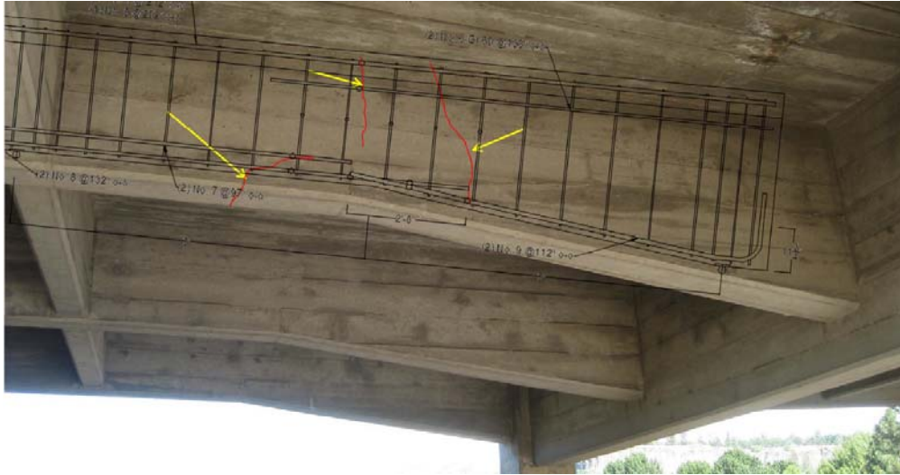
Figure F.4 – Rebar cage overlaying critical crack locations (ODOT, 2013)
