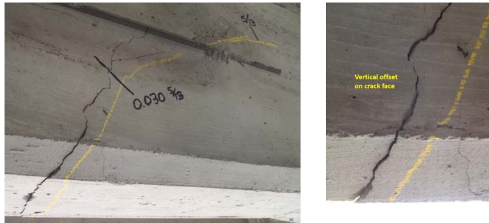
Figure F.2 – Vertical offset at crack interface (ODOT, 2013)
