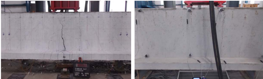
Figure A.82 – Specimen IT.0.0(6).Ti front and back failure photographs
