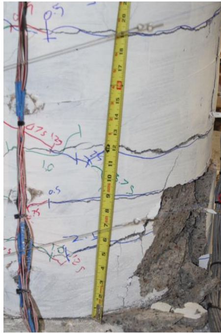
Figure 2.5 Photograph of column G80-1 crack mapping and concrete spalling
