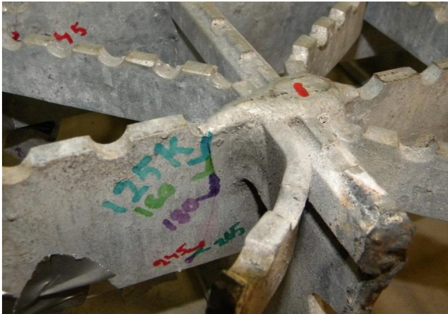
Figure 5.30: 'S' crack initiation from weld run off
