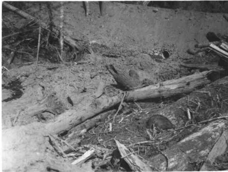
Figure 2. Road Culvert in Unit 1D Showing Outlet and Debris.
