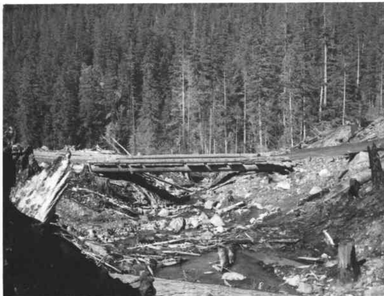
Figure 8. Same area as Figure 7 showing Extensive Flood Damage to road culvert.
