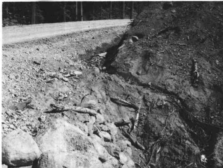
Figure 3. Road Drainage Entering Tributary in Unit 1D.
