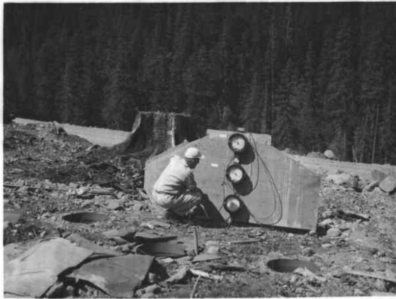
Figure 11. View of Experimental Temperature Apparatus.
