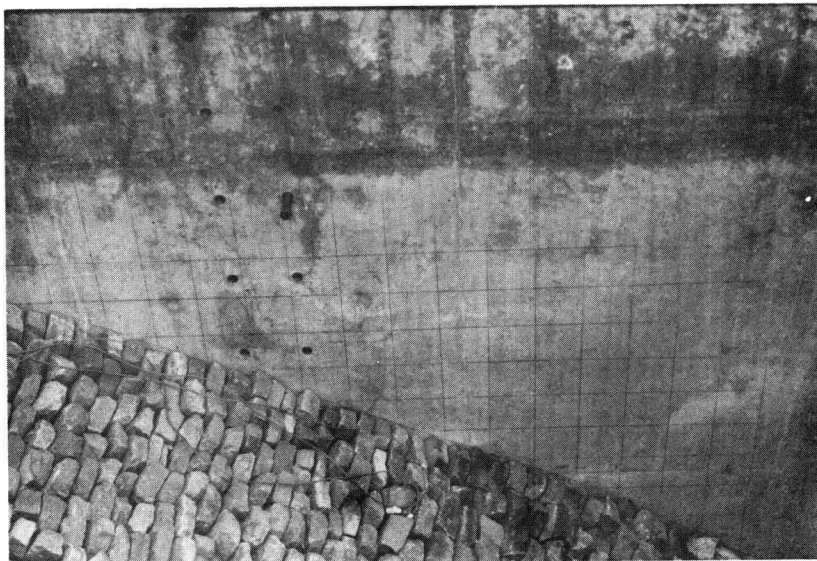
Fig. A-13. Grid Used to Measure Runup and Rundown
