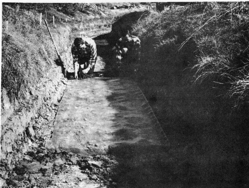
Figure 1. Placing the eight-mesh nylon screen in the bottom of the Prosser West Branch Canal.
