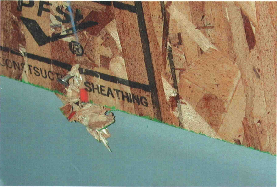
Figure 12. OSB sheathing edge breakout at the sill plate
