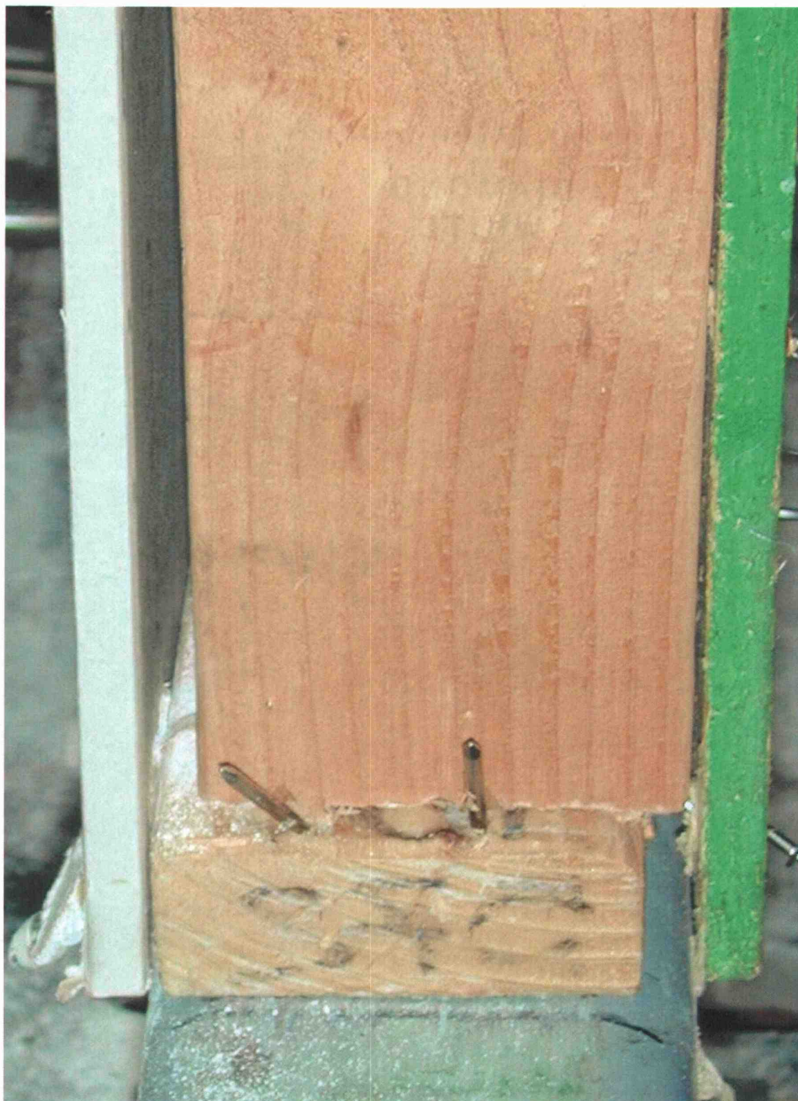
Figure 11. Uplift caused wall end stud to separate from the sill plate
