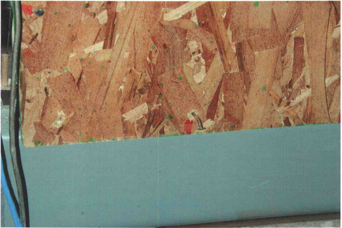
Figure 24. OSB sheathing nail withdrawal and nail pull-through along the sill plate
