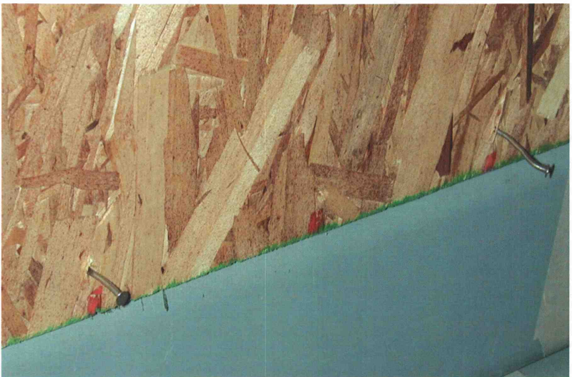
Figure 20. OSB sheathing nail withdrawal and nail pull-through along the sill plate
