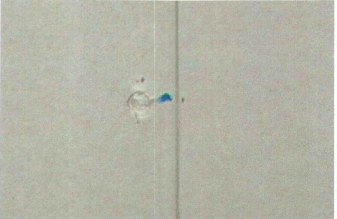
Figure 8. Localized crushing of the GWB panel along the center stud
