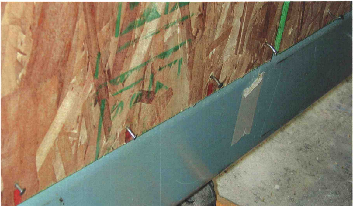
Figure 2. OSB sheathing nail withdrawal along the sill plate
