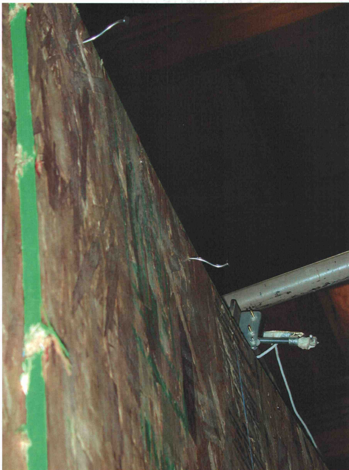
Figure 4. OSB sheathing nail withdrawal along the top plate (at top of picture) and OSB separation from the framing at the center stud (at left of picture)
