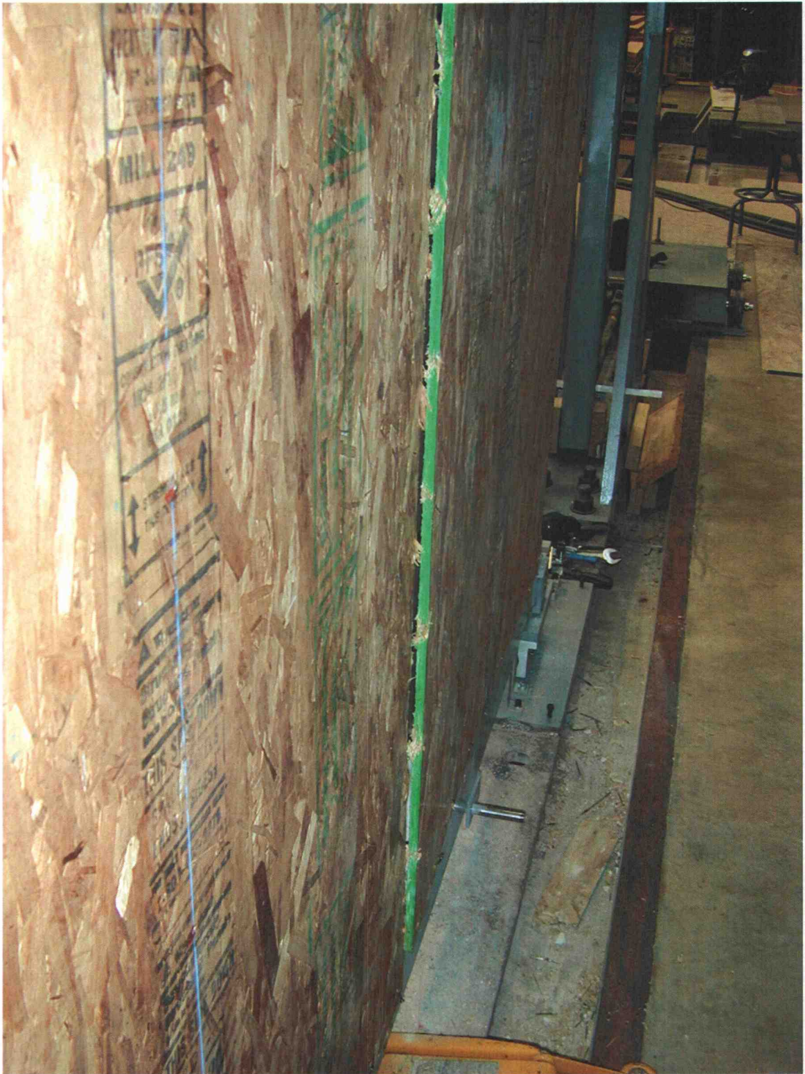
Figure 5. OSB separation from the framing along the center stud
