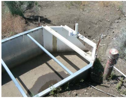
The ultrasonic sensor in Mays recorded no changes in depth of flow. Sediments on the flow of the flume are less than 31 mm (1/8 inch) deep.
