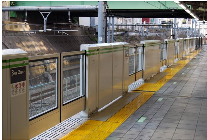
Figure 4: Half height platform doors at Meguro Station Tokyo, Japan
