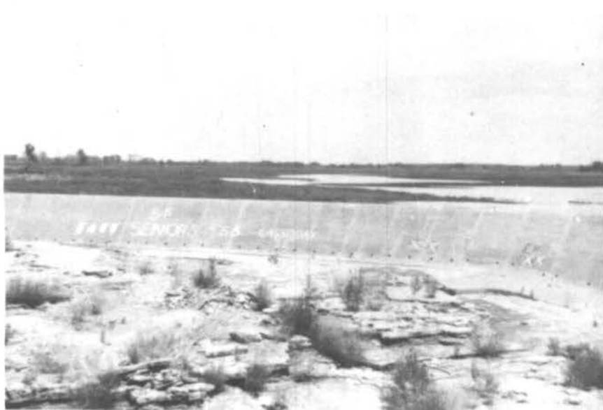
FIG. XIII. SILTATION HAS REDUCED VOLUME OF LAKES
