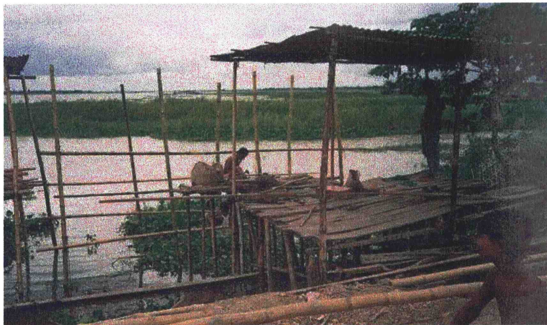
Figure 16. Temporary platforms being erected along the edge of an elevated road bed in Village 3.
