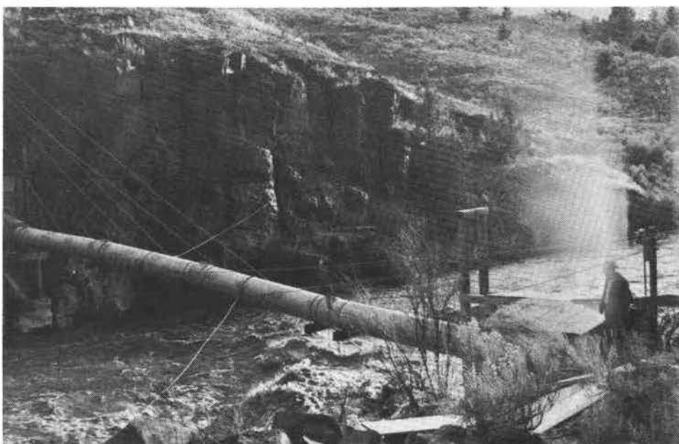
Figure 14 Irrigation structure across John Day River near Dayville, Oregon. Capacity 8 c.f.s.
