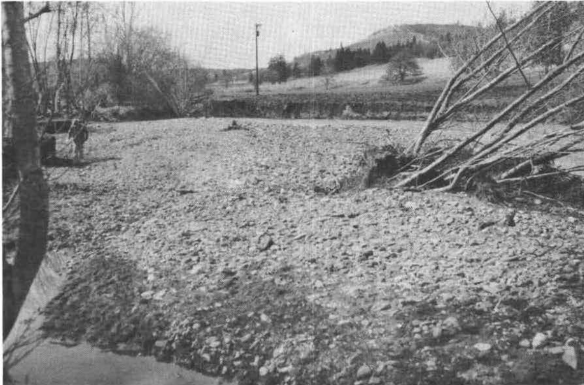
Photo 27.--A gravel and debris bar has almost filled the channel on Fifteenmile Creek during one flood which caused severe bank erosion, Oregon. SCS photo. NO. 7-1099-1
