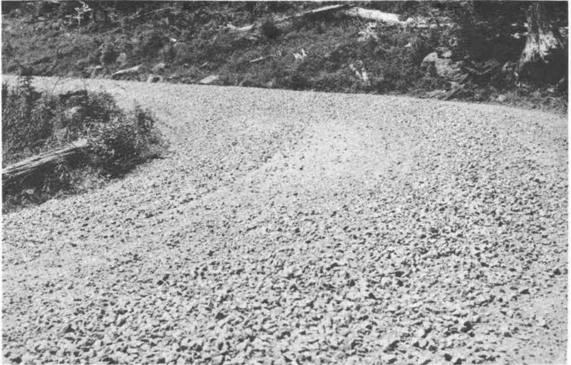
Photo 14.--Permanent forest roads should be surfaced with rock and graded with a center crown to provide for surface drainage. FS Mount Hood photo. 800. 8
