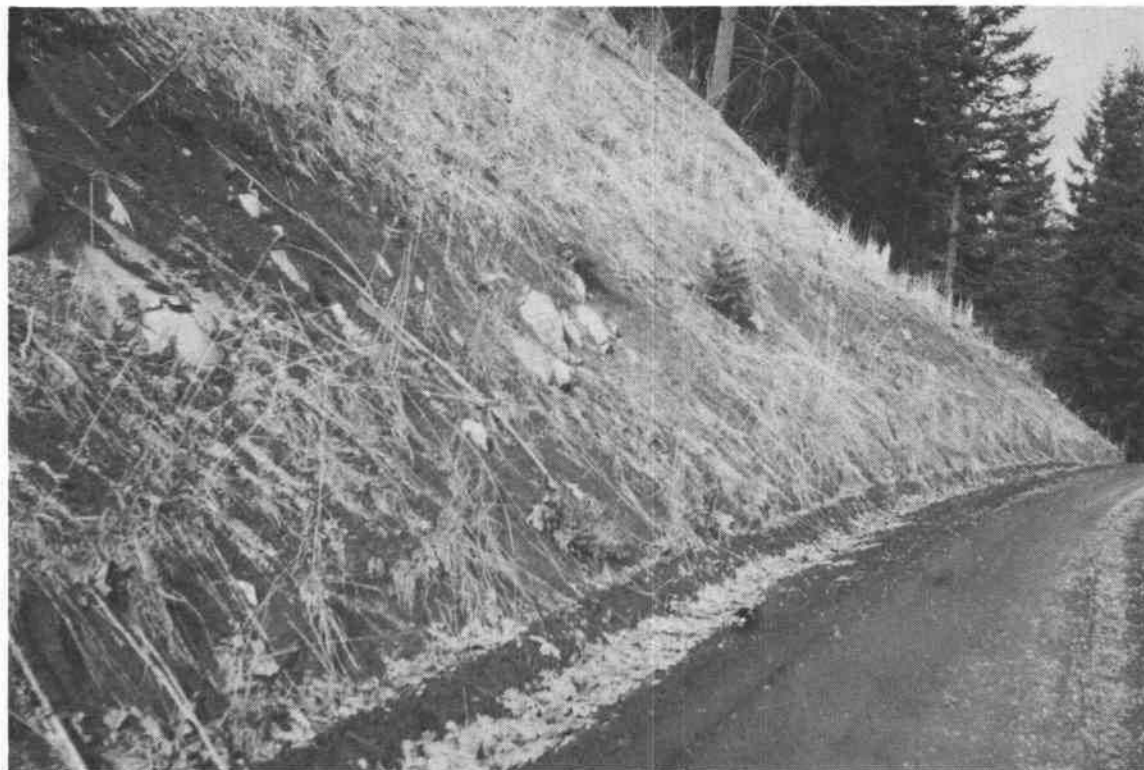
Photo 32.--Roadbank erosion control by vegetative methods on the Bear Creek road. FS Parkdale Ranger District photo. * * *
