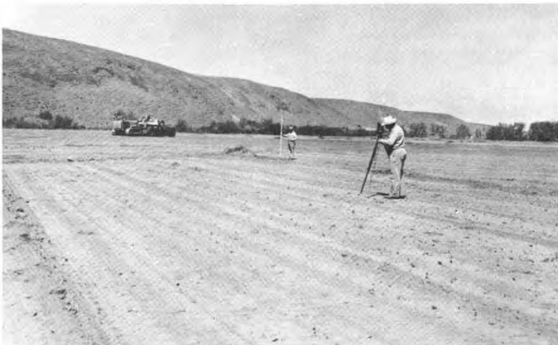
Figure 32.--Land is leveled for more efficient application of irrigation water, subbasin 3. SCS photo. 7-736-2
