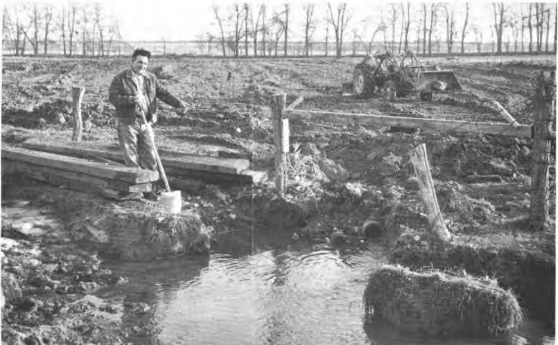
Figure 35.--Tile drainage system is newly installed to drain land in subbasin 2. SCS photo. 7-1077-7
