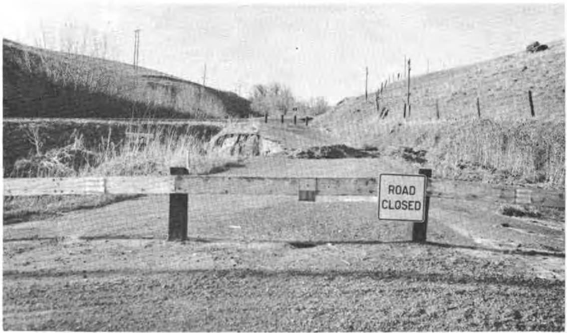
Figure 30.--The road is closed due to flood damage, sub-basin 2. SCS photo.
