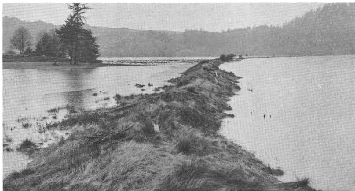
Photo 23.--Inadequate dikes and tidegates allow flooding along the Little Nestucca River in Oregon. SCS photo
