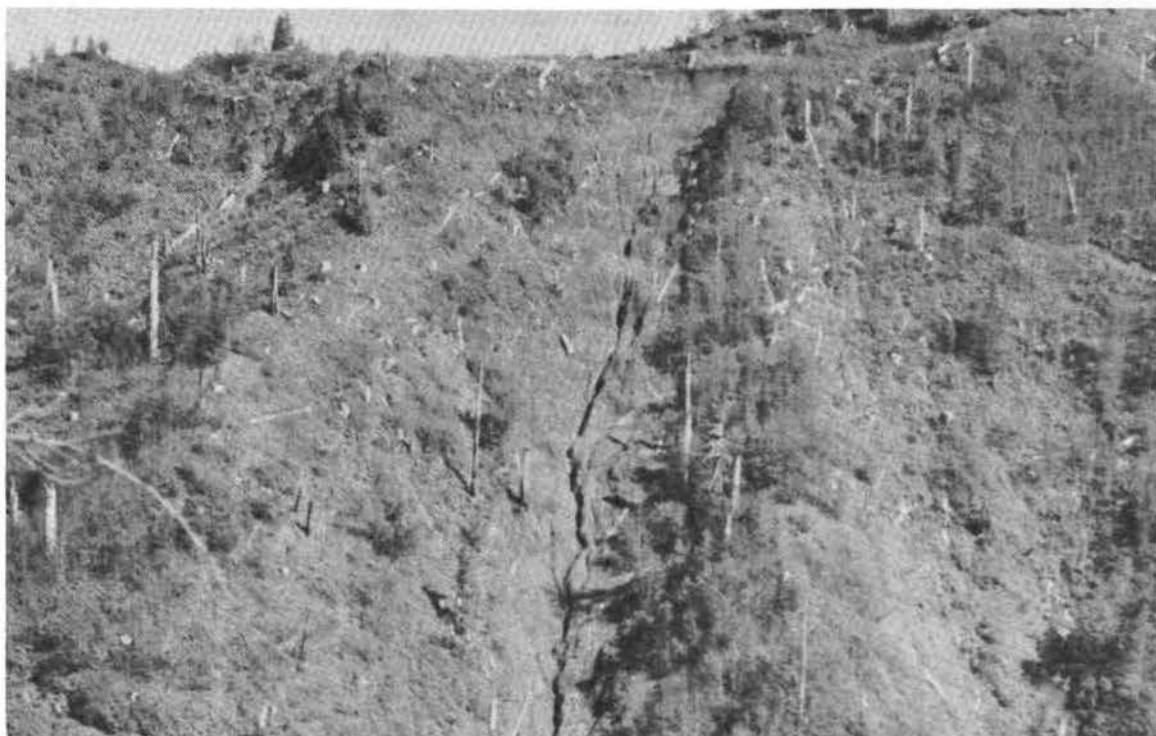
Photo 37.--This gully was caused by road construction near Anderson Creek in the Nehalem Subbasin in Tillamook County. FS photo
