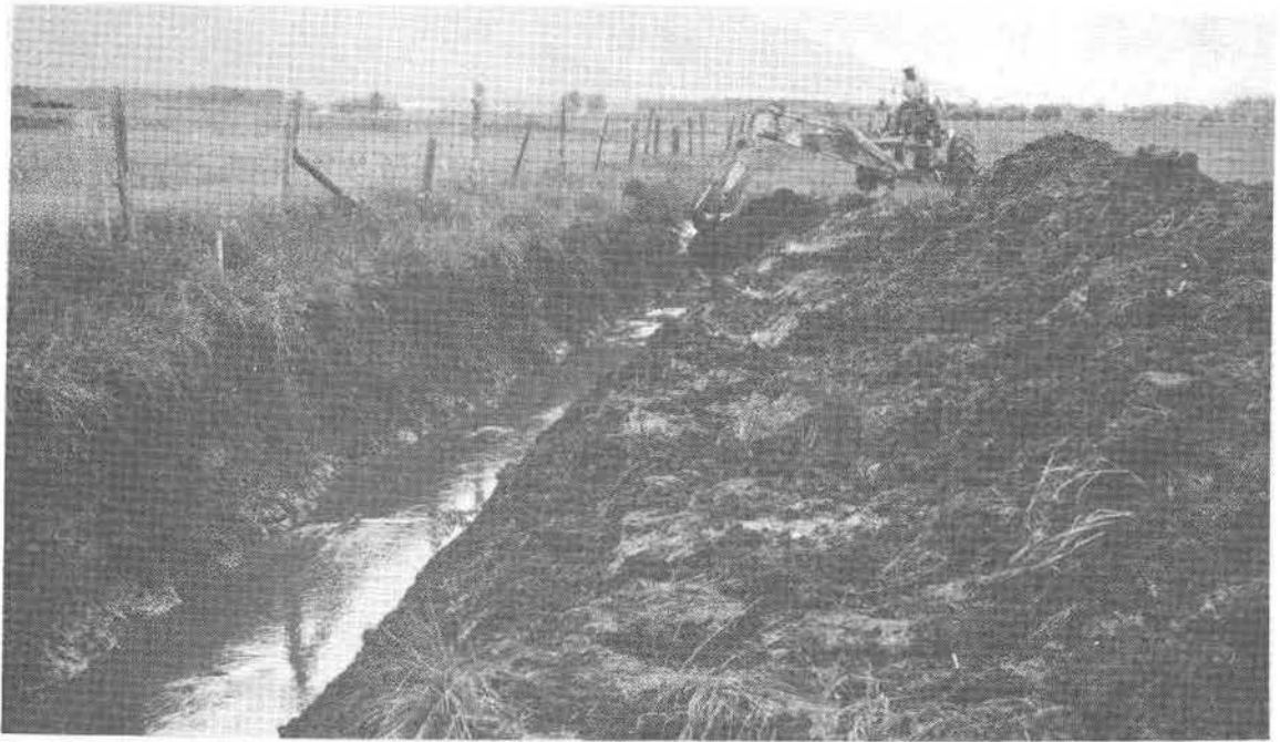
Photo 27.--This drainage ditch, under construction in the Baker Valley, will drain 30 acres that have been too wet for pasture or hay. SCS
