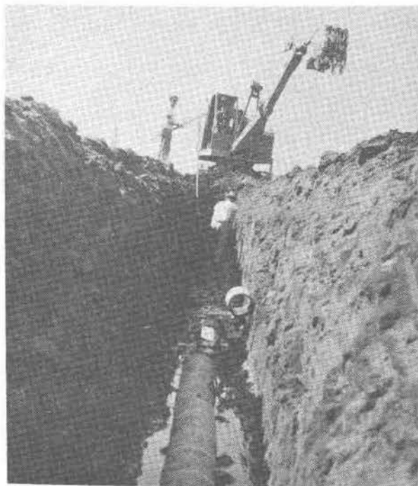
Photo 28.--This closed tile drain is under construction in the Baker Valley. SCS
