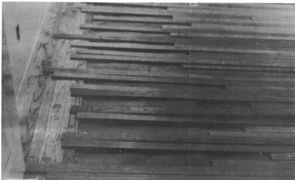
Figure 1. --Strip floor under construction in San Francisco area. Flooring is usually fitted in place over the entire area before it is nailed. Note border at the wall.
