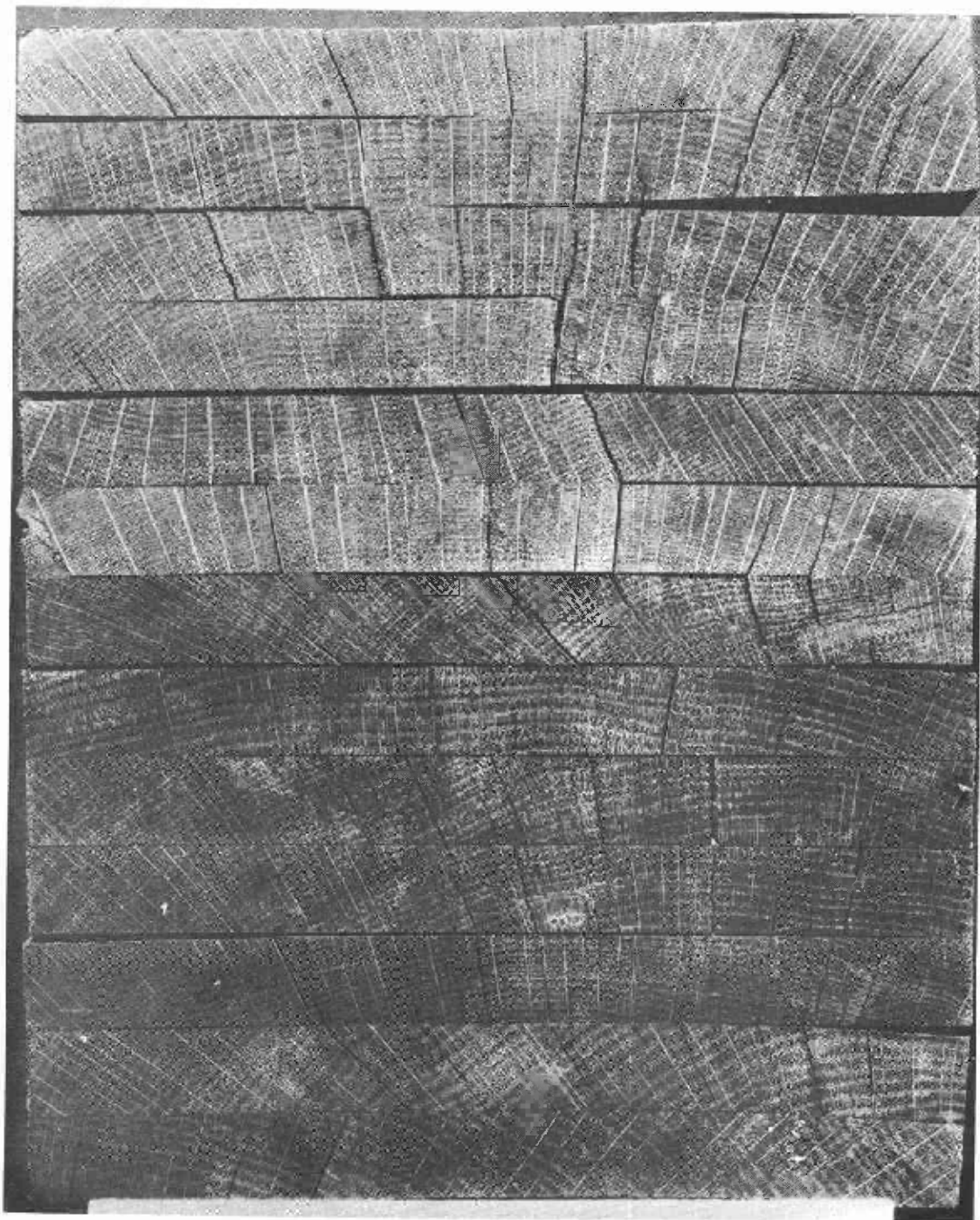
Figure 2.--Cross section of white oak beam, exposed to three cycles of the 30-day soaking -- 30-day drying test, indicates poor durability of glue joints.
