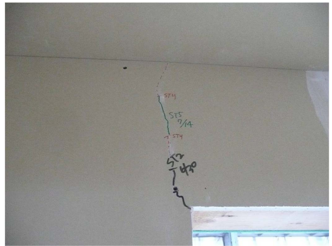
Fig. 19. Story 6, Wall E1; cracks develop all the way through panel after Seismic Test 5
