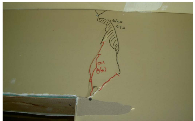
Fig. 9. Crack on Wall D1, Story 4 (over door opening) after Seismic Test 2
