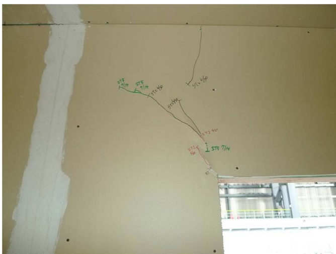
Fig. 18. Story 2, Wall E2; cracks failing to connect together after Seismic Test 5
