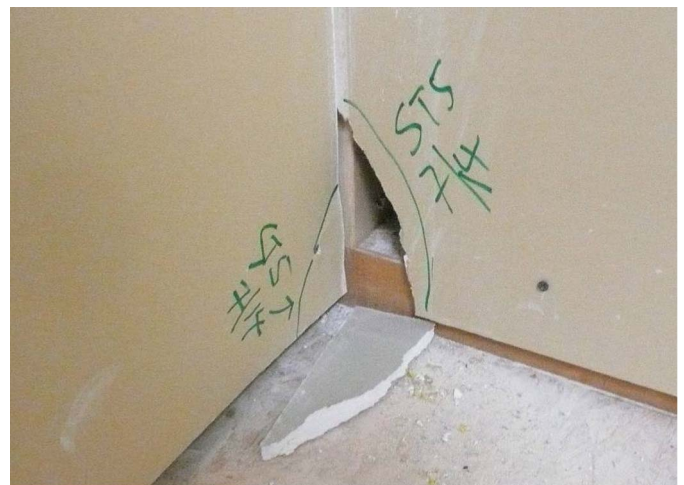
Fig. 15. Crack on Wall D2, Story 6 (corner crushing) after Seismic Test 5
