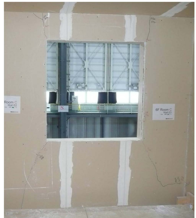
Fig. 20. Story 6, Wall E2; cracks develop all the way through panel for all corners after Seismic Test 5
