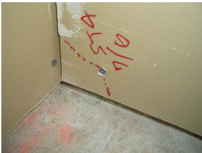
Fig. 12. New crack on Wall D1, Story 3 (corner crushing) after Seismic Test 4
