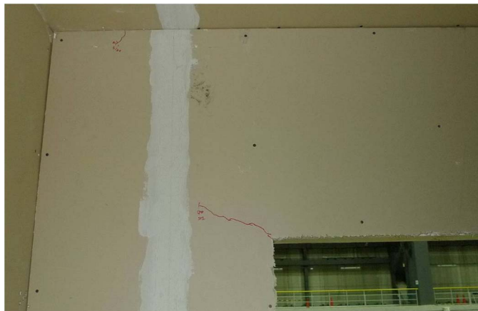
Fig. 8. Minor crack on Wall E4, Story 2 (over window opening) after Level 1 shaking
