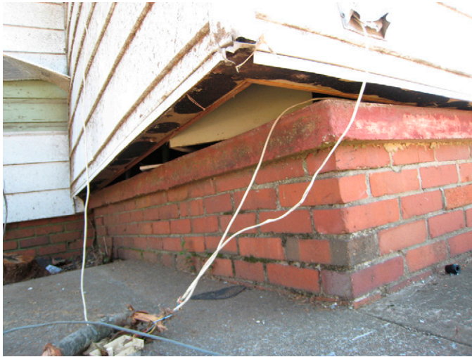
Fig. 9. Example of observed DOD5: building shifted off of the foundation
