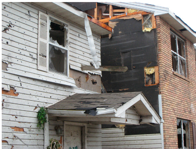
Fig. 7. Example of observed DOD3: broken windows
