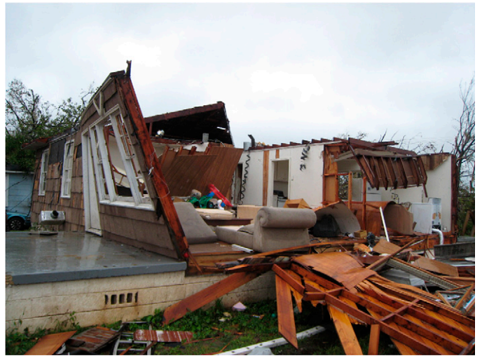
Fig. 11. Example of observed DOD7: exterior walls collapsed
