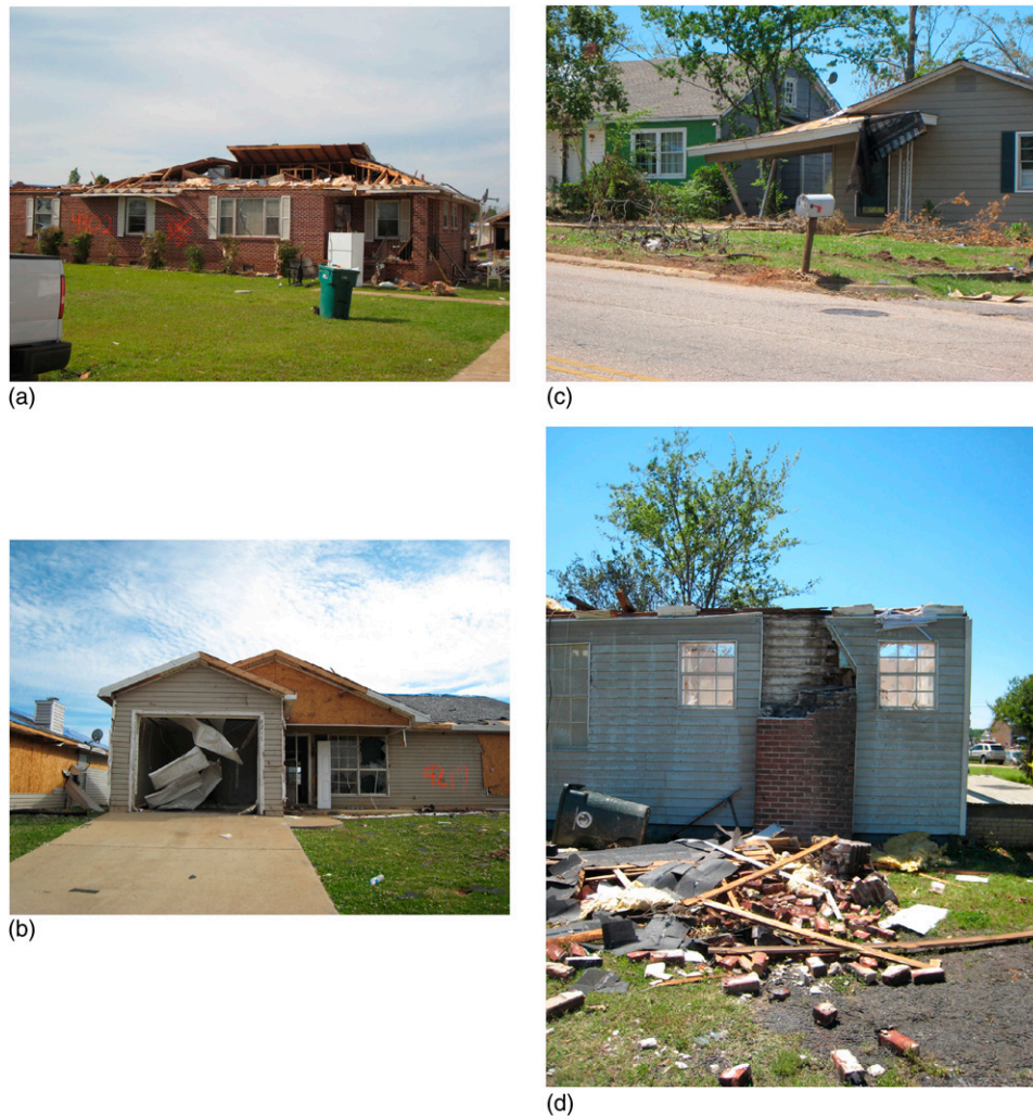
Fig. 8. Examples of observed DOD4: (a) significant roof damage; (b) garage door blown in; (c) porch damage; (d) chimney collapse
