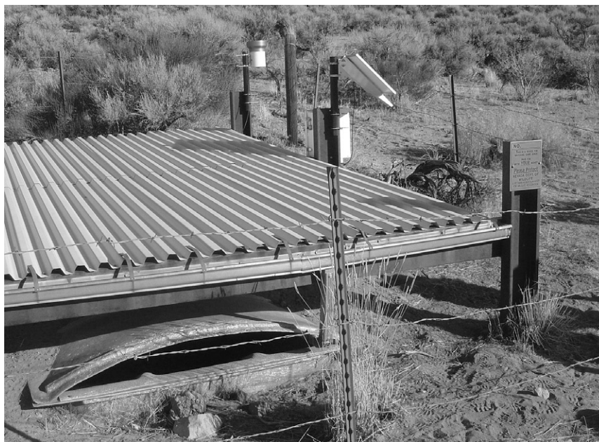
FIG. 3. Rain gauge, datalogger, and solar panel installation at Dry Valley No. 11 guzzler site.
