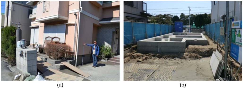
Figure 9. (a) Tilt and settlement of a residential home in Urayasu, and (b) foundation for a residential home in construction (GEER 2011).
