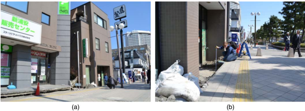
Figure 8. Differential settlements between a gray building on piles, a brown building on a shallow foundation (brown building on the right), and the ground surface in Urayasu (GEER 2011).
