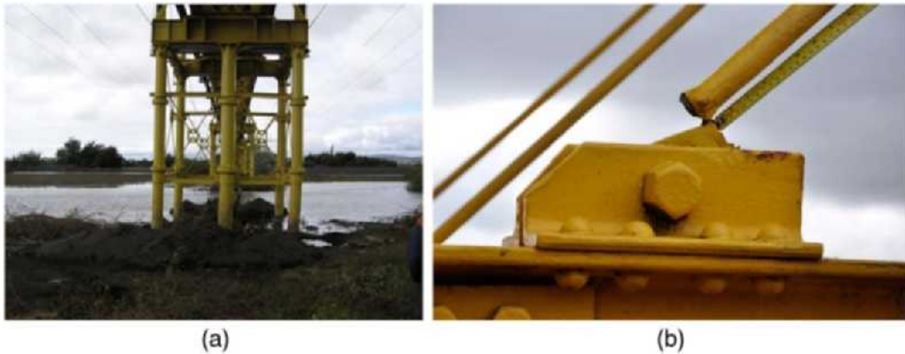
Figure 24. Bio-Bio River railroad bridge: (a) Pillars translated and rotated during earthquake; (b) detail of broken crossbar, S36.836075° W73.086969°.
