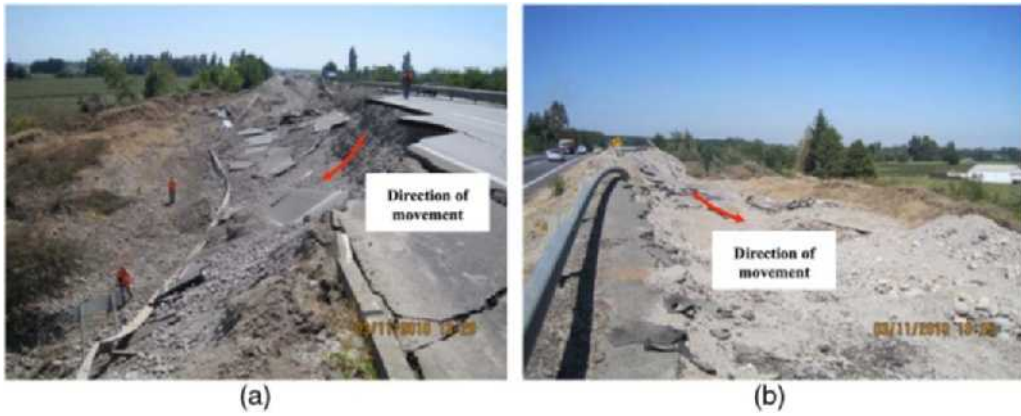
Figure 18. Embankment fill collapsed near Copihue, north of Parral, closing the southbound lanes of Ruta 5: (a) view from the south, (b) view from the north, S36.087891° W71.791513°.
