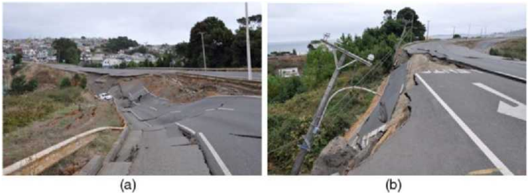
Figure 22. (a) View looking south on route 160 showing north bound failure area, S37.0730° W73.1475°; and (b) view looking north showing south bound failure area, S37.0746° W73.1479°.
