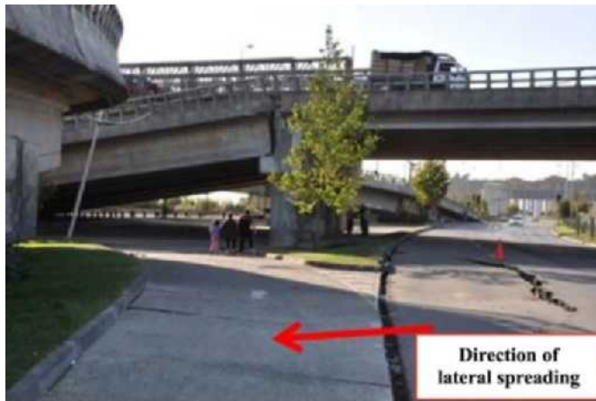
Figure 4. Deck unseating at Llacolén Bridge in Concepción. Cracking resulting from lateral spreading is visible on right side of photo. View north ( S36.830380^{\circ} W73.067541^{\circ} ).
