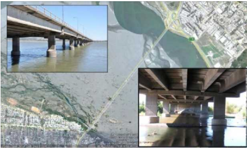
Figure 8. Juan Pablo II Bridge connecting the cities of Concepción and San Pedro de la Paz across the Bío-Bío River. Typical bridge bent configuration shown in photograph inset.
