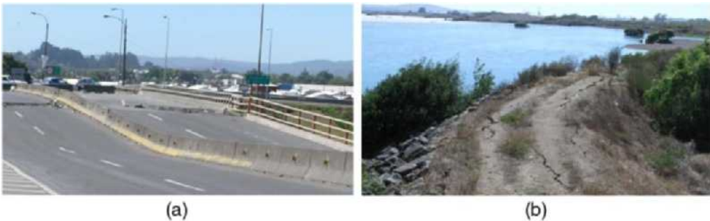
Figure 9. Juan Pablo II northeast approach: (a) Settlement of bridge deck near bridge approach (view East, S36.815900° W73.084064°); (b) lateral spreading of northeast approach embankment.
