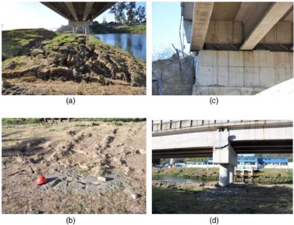
Figure 16. Liquefaction-induced damage at La Mochita bridge: (a) Looking north at bent #3, S36.847389° W73.055219°; (b) sand boils observed below the bridge, S36.847456° W73.055129°; (c) transverse shift of deck relative to south abutment, S36.847547° W73.054876°; and (d) damage to transverse shear key at bent #3, S36.847405° W73.055084°.
