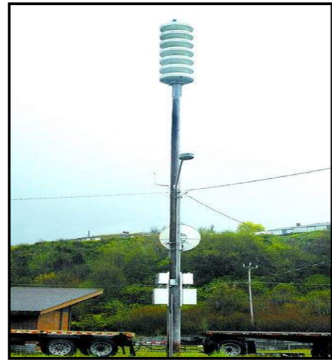
Figure 11: Tsunami Warning Siren
