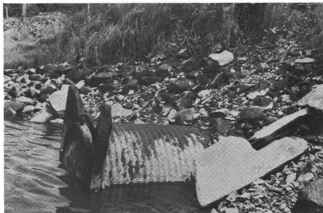
Dikes and Flood Gates Protect Clatsop Farm Lands
