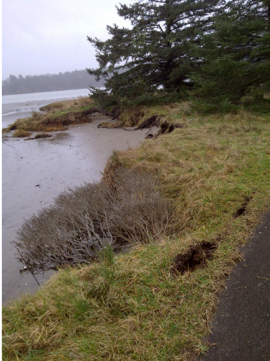
Figure 4.4: View to the south of the 2011 DRP in the Reference area (February 14, 2013), showing collapsed banks with 4 foot vertical scarps. In the upper left, erosion is now starting to attach low salt marsh habitat on the point and beyond which has not previously been exposed to erosion.
