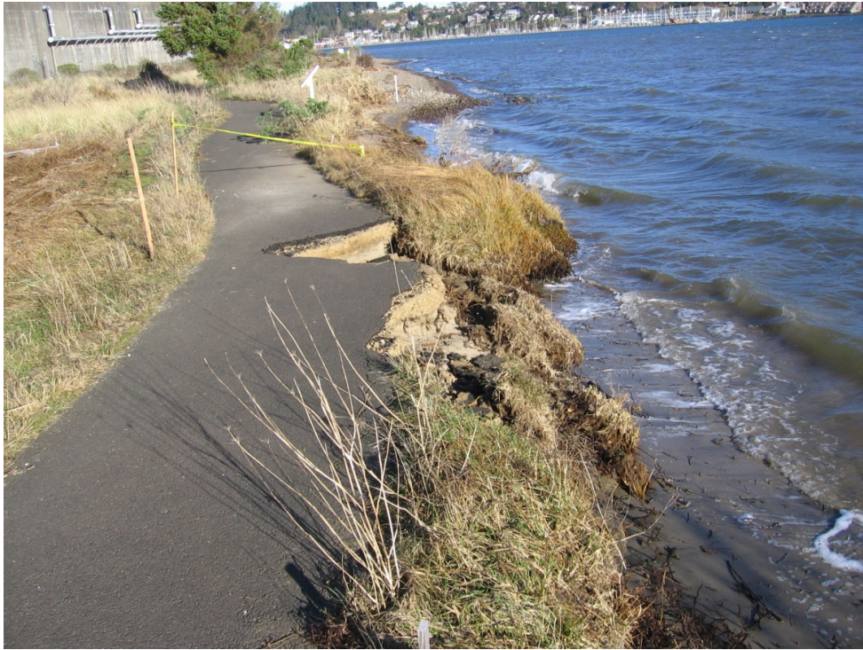
Figure 4.1: View of collapsed section of HMSC nature trail, February 3, 2012.
