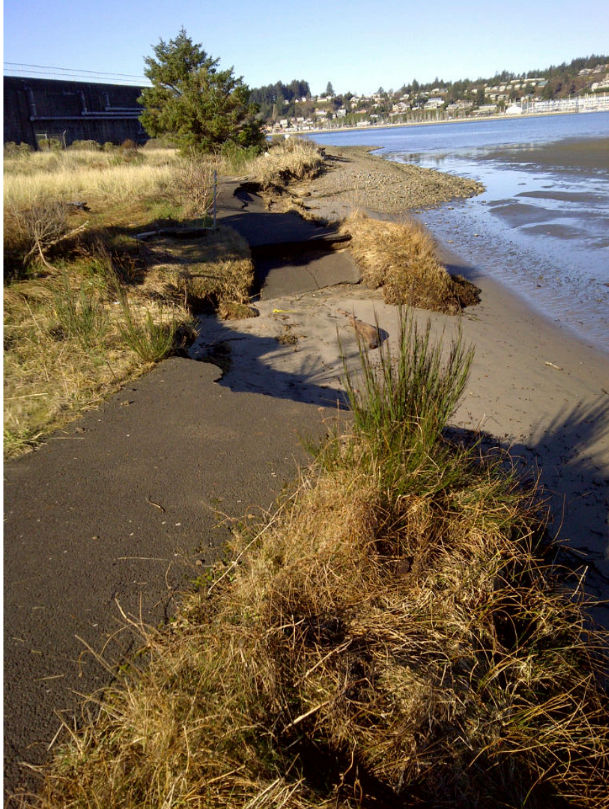
Figure 4.2: View of collapsed section of HMSC nature trail, January 16, 2013. The trail has been completely washed out in the foreground. The trail information sign seen at the top of Figure 4.1 has been removed after erosion undermined the posts supporting it. An additional 60 feet of trail in the middle distance has been undermined and the asphalt has collapsed on the shore.
