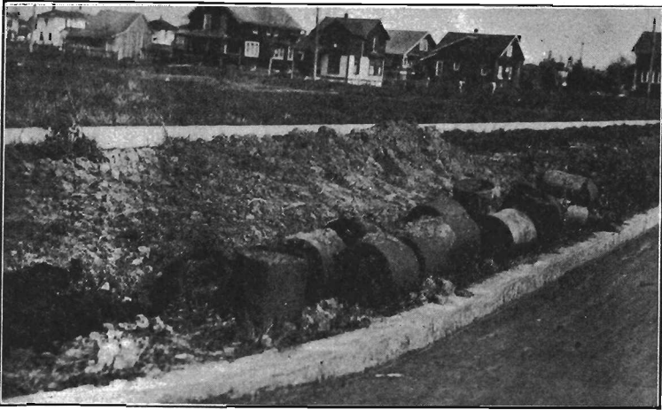
Figure 29. Tile Silted. Due to Poor Outlet.
