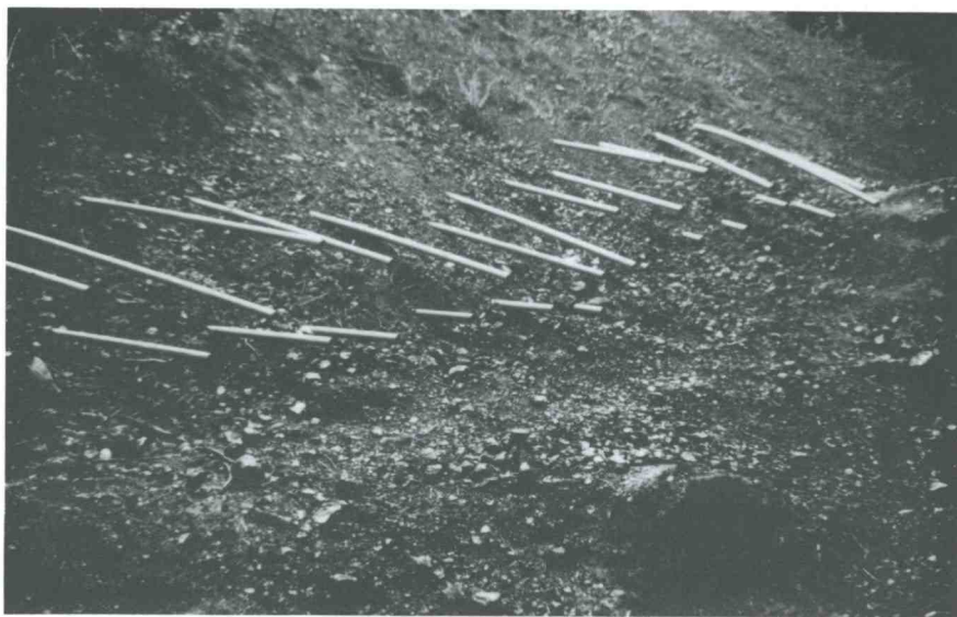
Figure 11. Perforated horizontal drains installed into road cuts and fills can reduce the chance of deep-seated slope failure.
