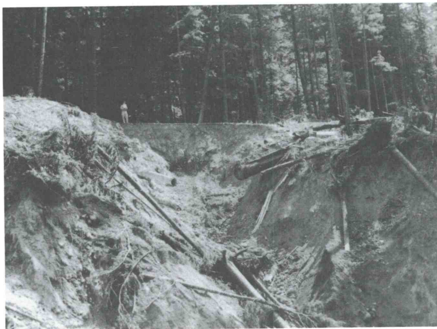
Figure 9. Poor road drainage can result in catastrophic fill-slope failures.
