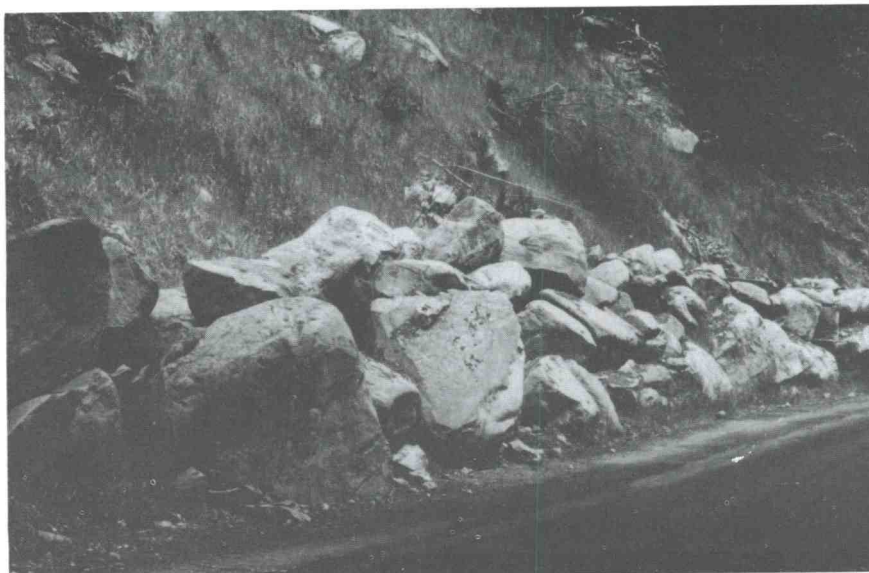
Figure 12. Rock buttresses can control localized slumping along road cuts.
