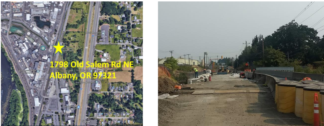
Figure 4.6 Study site, Truax Creek Bridge in Albany, OR. Left: Google Maps showing the location of the bridge. Right: Photo showing the southbound lane near its completion date.
