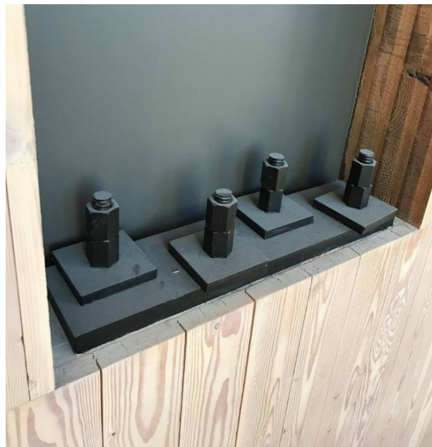
Figure 2.2. Tensioned rods secured by hex nuts protruding out of CLT shear walls at Peavy Hall, Oregon, USA.
