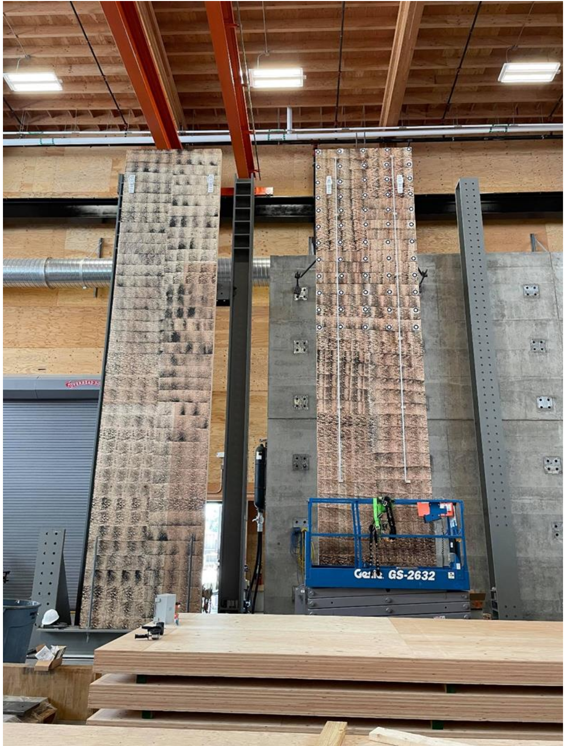
Figure 4.9. Erected MPP (left) and CLT (right) walls during instrumentation of rods, LVDTs, and targets
