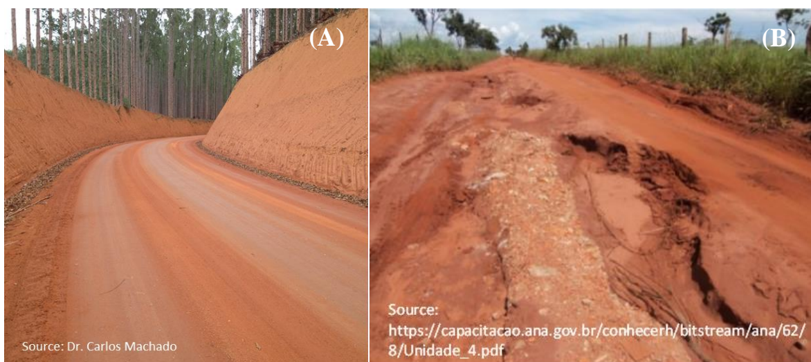
Figure 2 – Conditions of unsealed road in Brazil. (A) demonstrate a state-of-the-art unsealed road properly built and maintained. This specific road was built with cement as the chemical stabilizer (Source: personal archive from Dr. Carlos Machado). (B) unsealed road with poor maintenance conditions, highlighting the erosion at advanced stages. The loose material will be carried to the closest water body by rain oof or as dust emissions by traffic (Source: https://capacitacao.ana.gov.br/conhecercerh/bitstream/ana/62/8/Unidade_4.pdf ).
