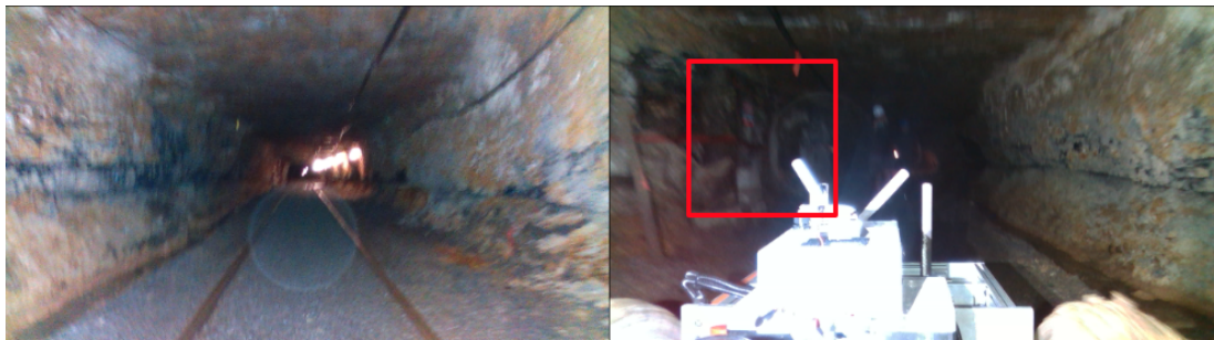
(a) Left: Forward facing image. Right: Backwards facing image with vertical brace structure in red box, not visible due to lack of light.
