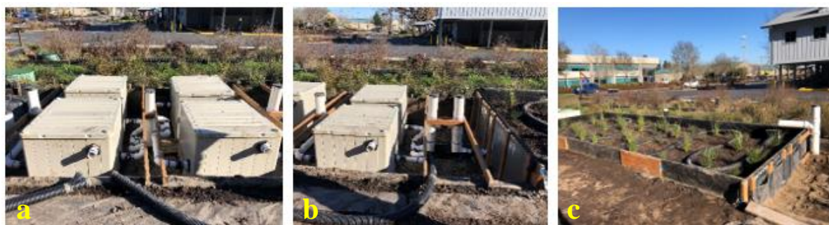
Figure 3.5 Photos of completed treatment train. Note: water flows start at the riser in image c and end at the far left riser in image a. (a) Sorbent boxes with risers 4 and 5. Biochar socks are in the right bins and RemBind® are in the left bins. (b) Outlet of LID with risers 2 and 3 connecting to the biochar sorbent boxes. (c) Vegetated LID with perforated hose and inlet riser 1.
