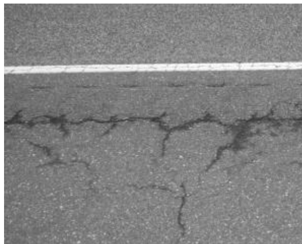
Figure 2.9: Fatigue cracking at milled rumble strips (Coffey and Park, 2016)
