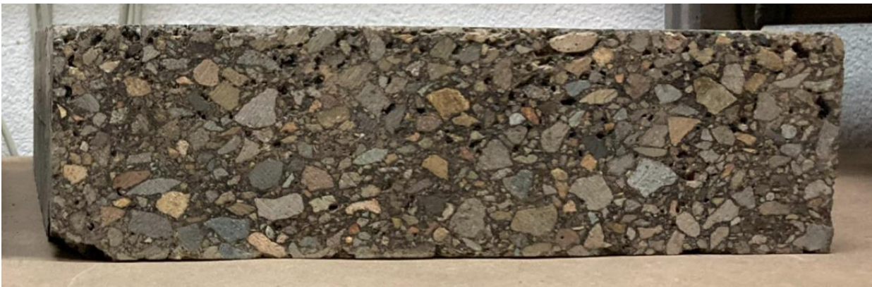
(b) Air voids – Unconstrained edge of travel lane
