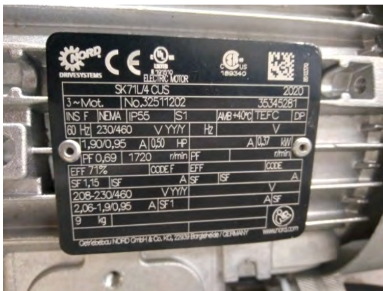
Figure 5.11: Nord gear motor nameplate.
