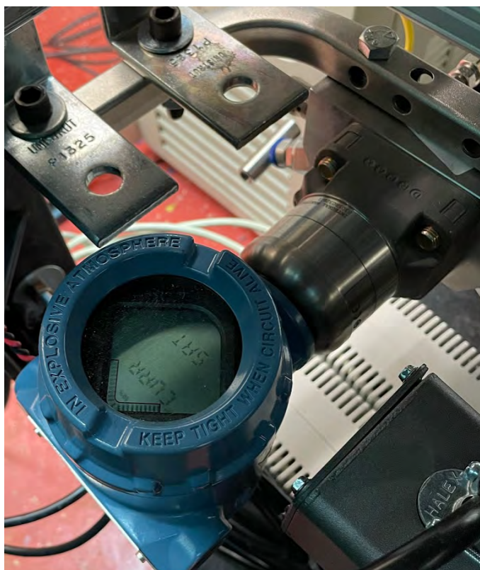
Figure 5.20: The Rosemount 3051SMV pressure transducer mounted on the test loop.
