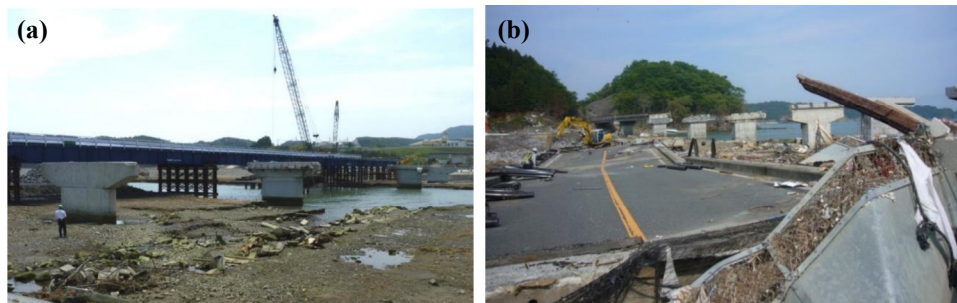
Figure 1. Damaged bridges after the 2011 Great East Japan Earthquake: (a) Koizumi bridge on the left (photo: E. Monzon) and (b) Utatsu Bridge on the right (photo: I. G. Buckle).
