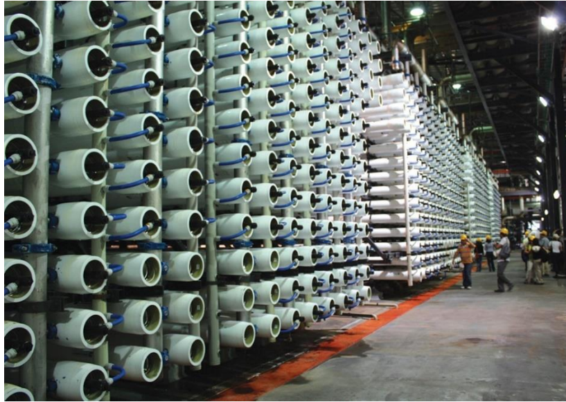
Figure 1-2. A full-scale desalination plant, featuring spiral wound membranes connected in series to form larger units called membrane trains. Fortunately, membrane trains are designed to be modular, so a single train can come offline for cleaning while the rest of the plant continues to operate (Dr. Sergio Salinas).
