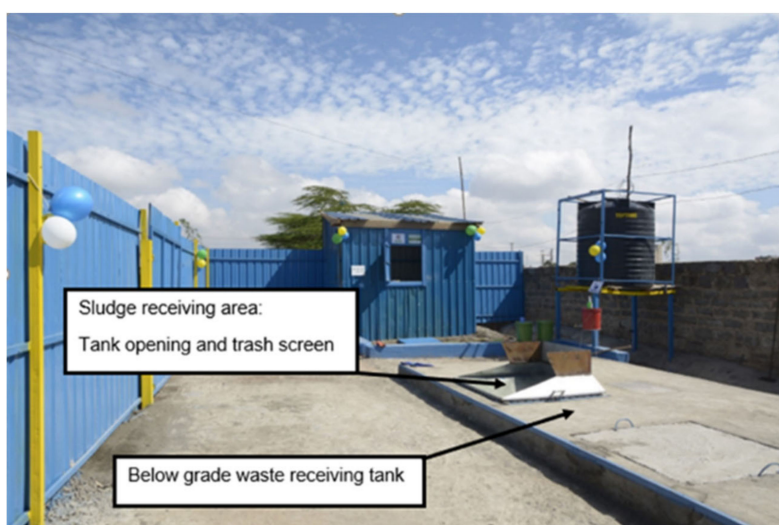
Figure 1. The Mtaa Fresh site contains a below grade tank in which pit latrine sludge is received from manual pit emptiers in Mukuru Kwa Njenga in Nairobi, Kenya. FS is delivered to the site in barrels. The contents of the barrels are tipped through a trash screen and into the tank. Photo Credit: Sanergy.
