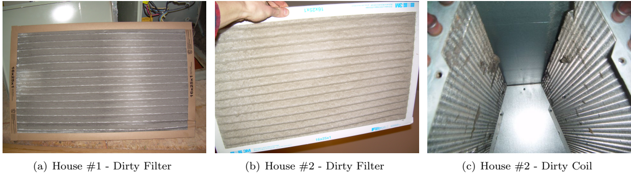
Figure 4.11: Photographs of Fouled Components
