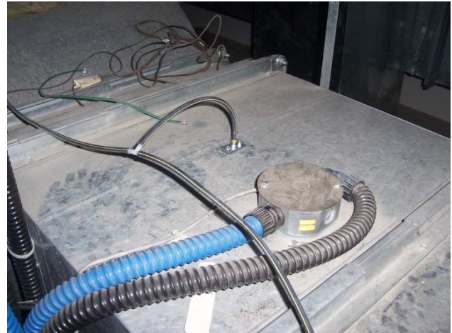
Figure 6: Installed Probe of Pressure Sensor
