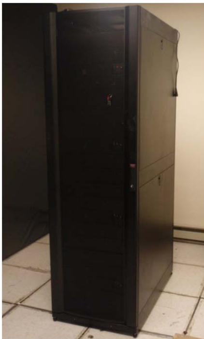
Figure 3–17: Rack with Server Simulators (Front View)
