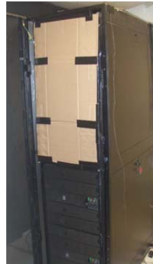
Figure 3–39: Top Servers Off and Blocked
