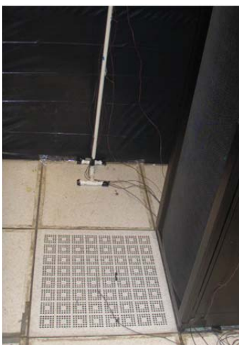
Figure 3–41: Rack Against the Perforated Floor Tile
