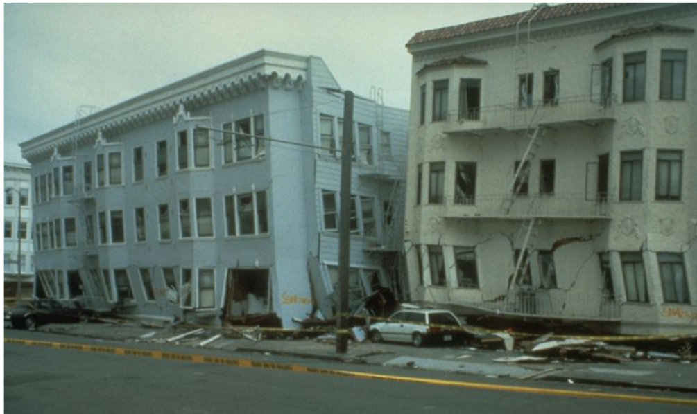
Figure 4.1 - Two multi-unit, wood-frame soft-story buildings that collapsed in the Marina District during the 1989 Loma Prieta earthquake. (ATC, 2009: Image courtesy of the National Information Service for Earthquake Engineering, University of California, Berkeley)
