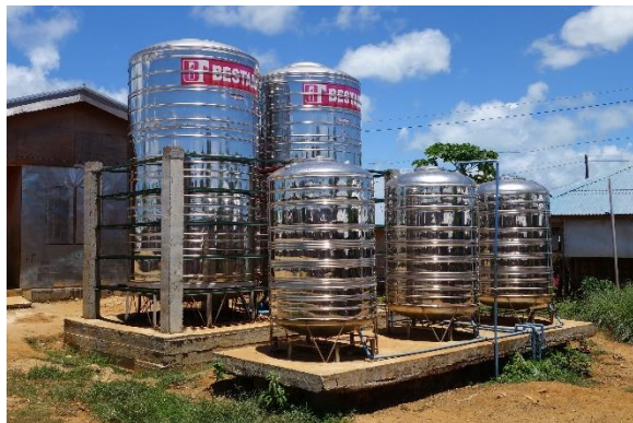
The site water storage and pump system that has gone unused.
