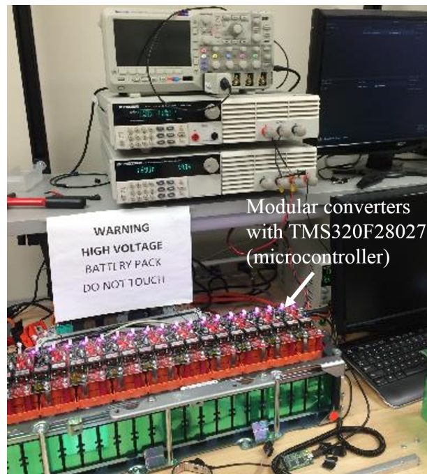
Figure 4.4: 21-cell battery pack at Utah Power Electronics Lab, Utah State University.
