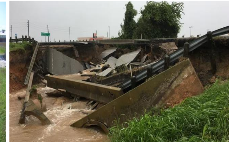
Collapse a bridge near Rosenberg, Texas during Hurricane Harvey, Source: [6]
