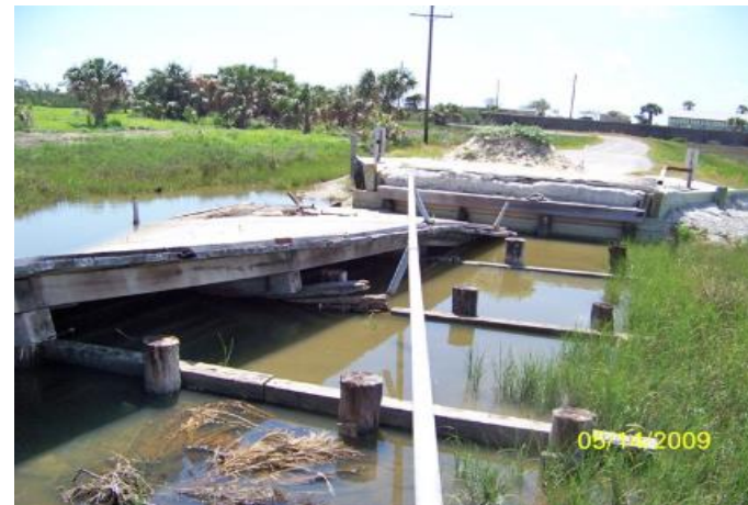
Damage of 7 th street bridge at Port Bolivar during Hurricane Ike, Source: [5]
