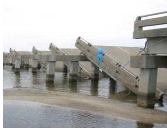
Damage of US-90 during Hurricane Katrina, Source: [3]
