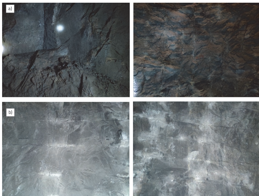
Figure 19. Excavation contour effect of controlled conventional blasting and controlled shaped-charge blasting: a) Excavation contour surface produced using controlled conventional blasting; b) Excavation contour surface produced by controlled shaped-charge blasting
