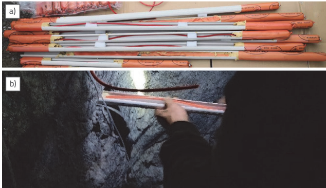
Figure 17. Charging and installation of shaped-charge tube on site: a) Charging of shaped-charge tubes; b) Site installation
