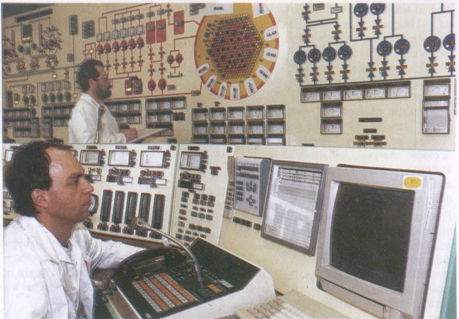
Control room of the Budapest Research Reactor
